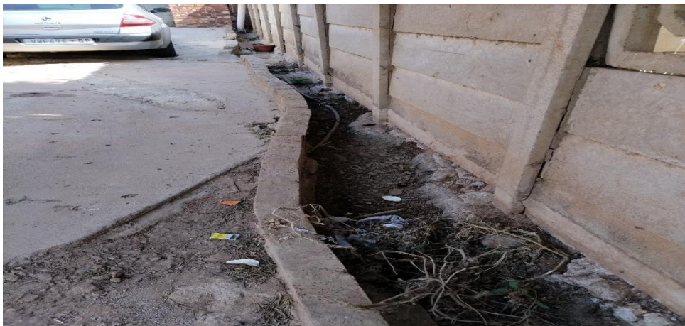
Figure 3: Dry furrow constructed by the Complainant's family to manage the outflow of the sewage spillage onto the street
