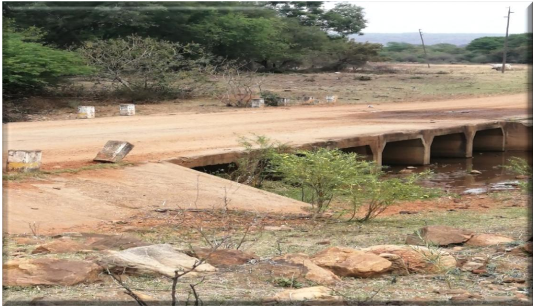
Figure 2: Bridge on road Z456, constructed to allow waterflow from the nearby Sehujwana dam
