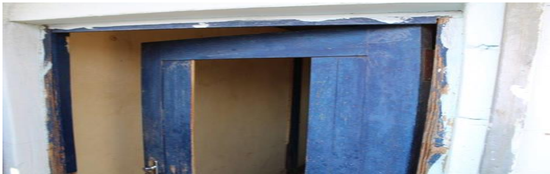
Figure 18: ablution facilities with broken doors
