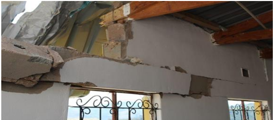
Figure 4: Uninhabitable classes damaged by the storm
