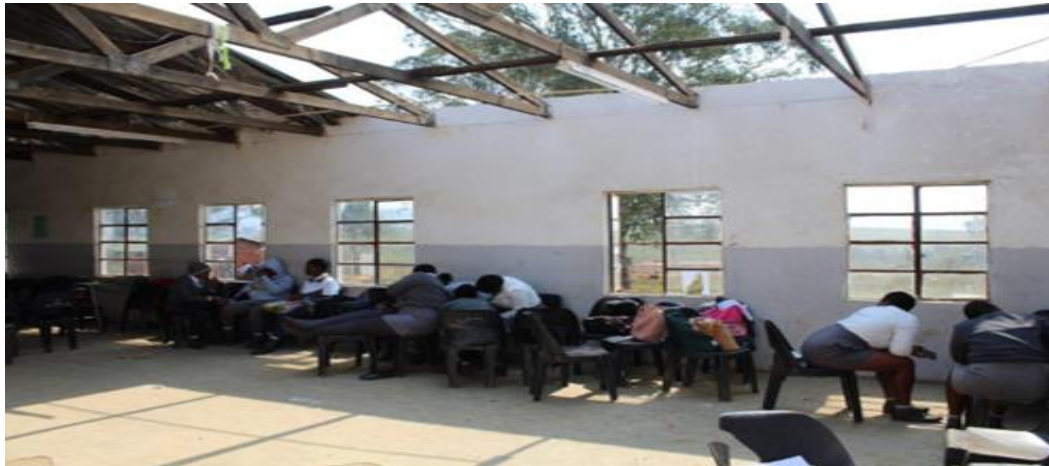
Figure 9: Classrooms with broken windows and doors
