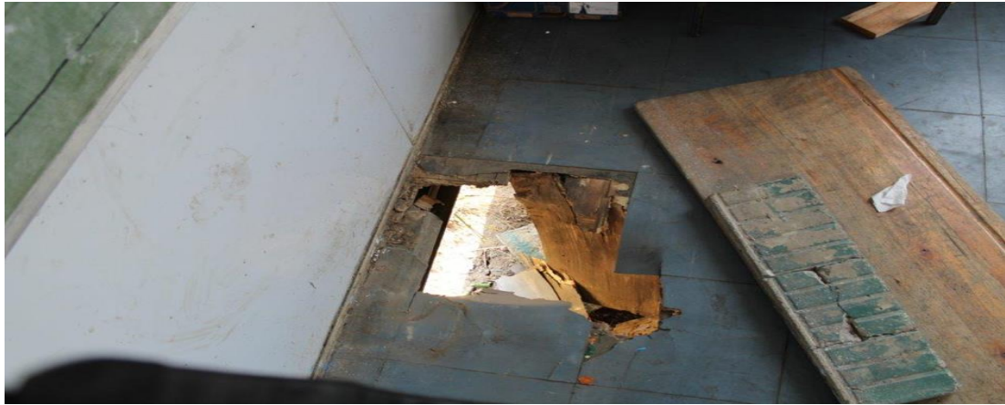
Figure 13: deteriorating mobile classrooms floors
