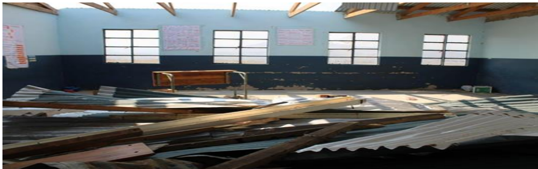
Figure 12: Damaged of classrooms
