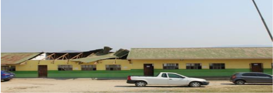
Figure 5: Partially damaged classrooms
