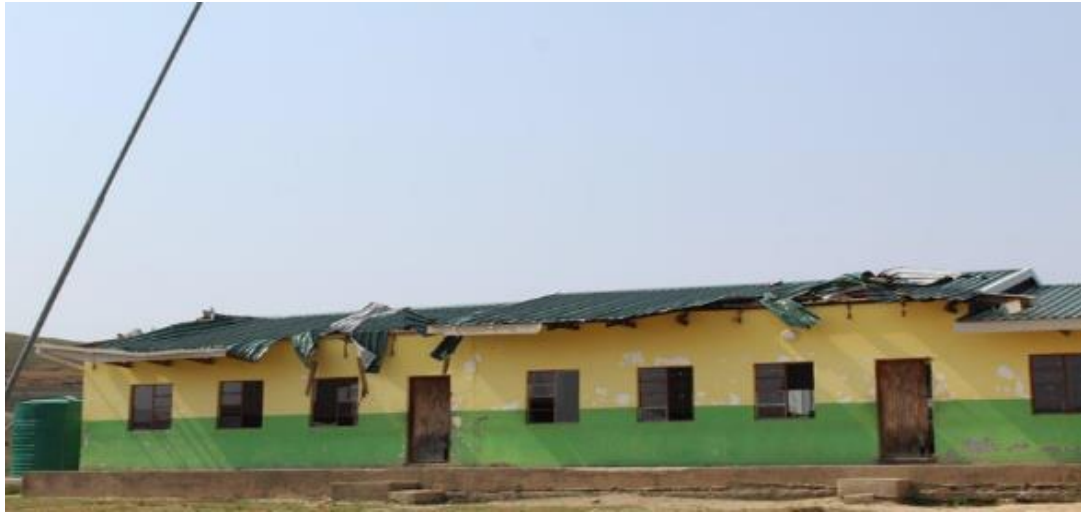
Figure 3: Uninhabitable classes damaged by the storm
