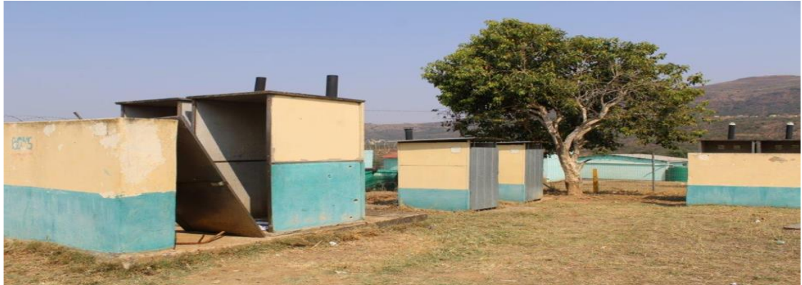
Figure 15: Ablution facilities in poor condition
