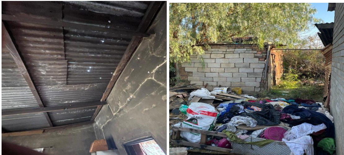
Figure 1: Burnt down dilapidated house (before construction)
